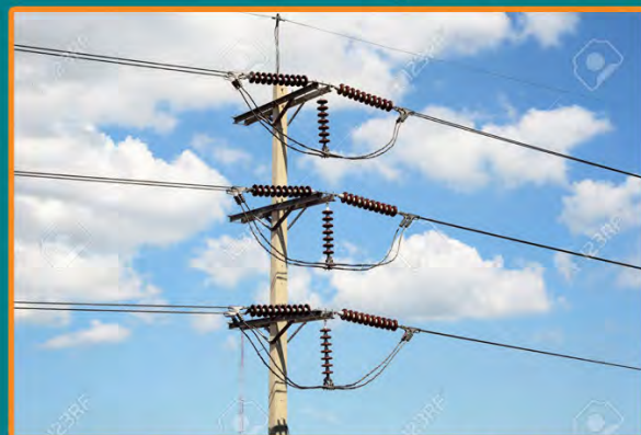
Line Constraction 13.2 KV & 69KV
